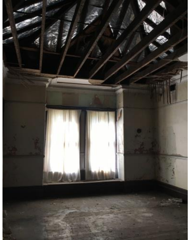
PICTURE 12 – INTERNAL VIEW SHOWING DILAPIDATED CEILING.
