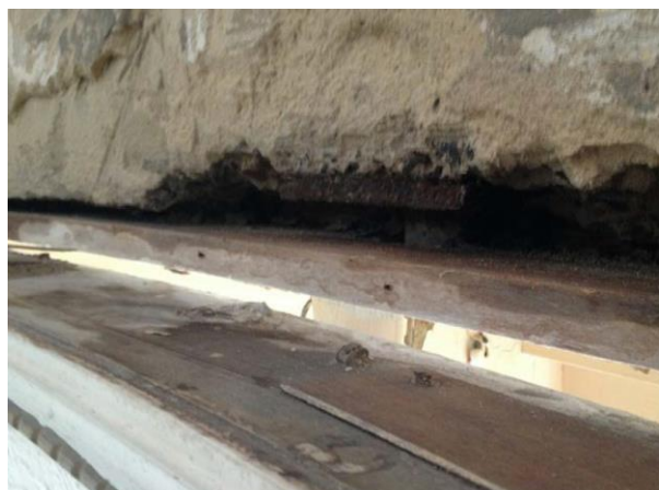
PICTURE 24 – DETAIL SHOWING CONCRETE CANCER
